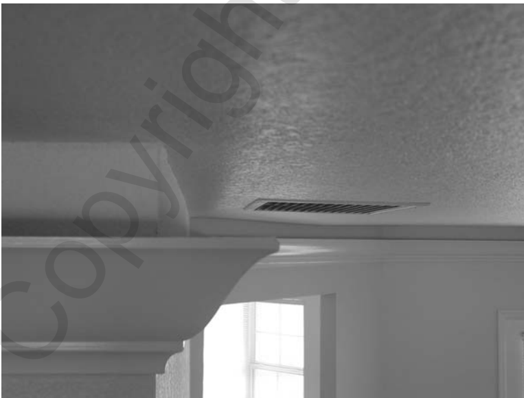
Figure 2.2 Dropped crown molding in the Gator Tech house for cabling and sensors.
